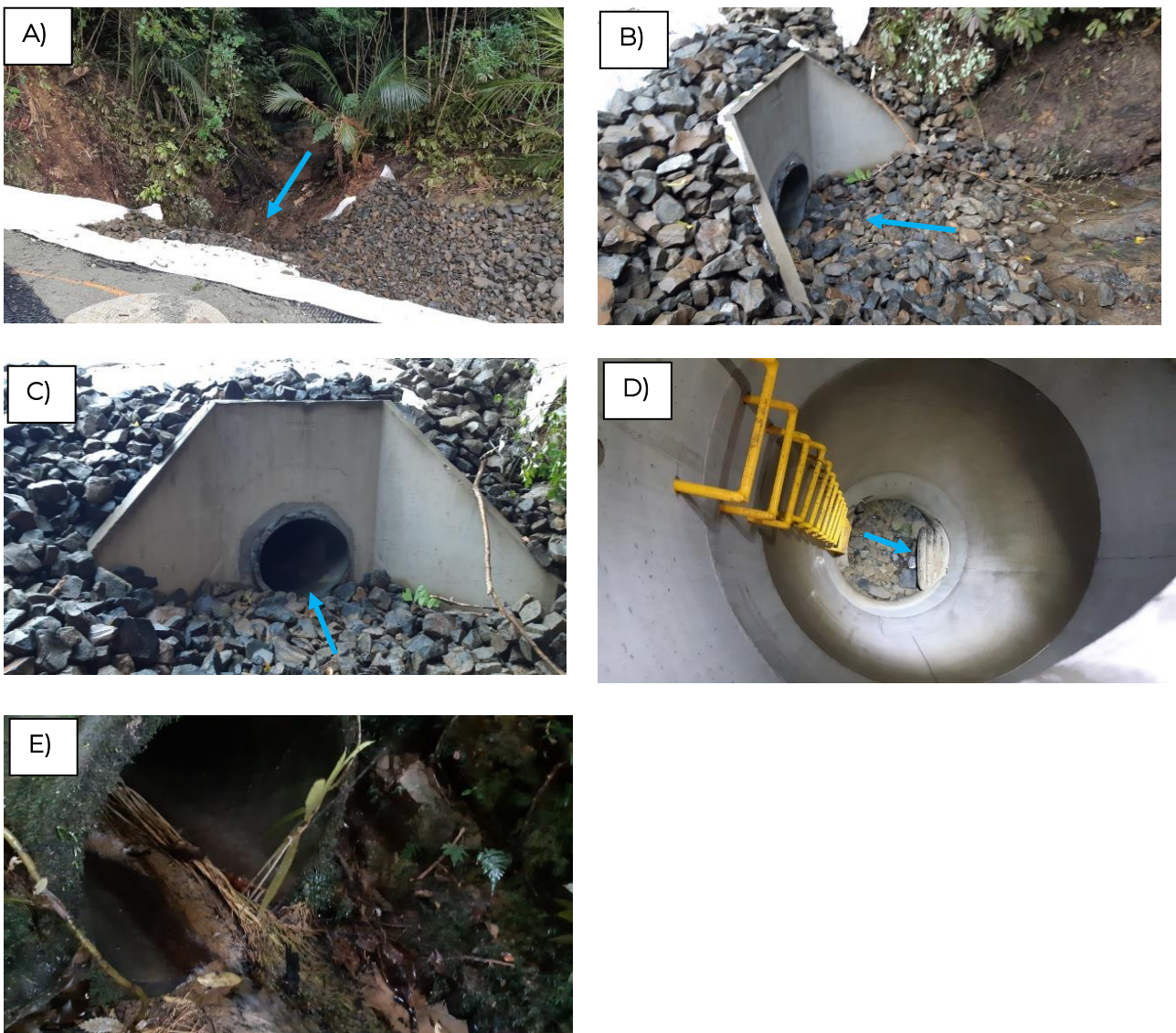
Figure A4. Site H: A/B/C) culvert extension and rip rap installed at inlet, D) manhole inlet currently still perched, E) outlet downstream of road.
