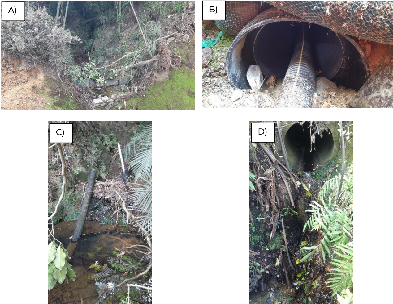
Figure A6. Site J: A/C) existing upstream stream habitat, B) newly installed emergency overflow at inlet that is offline to the main stream bed, D) perched outlet.
