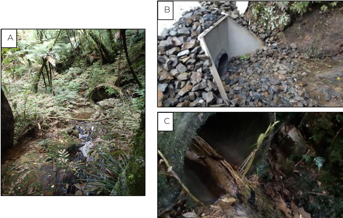
Plate 3-8: A) Stream at Site H, downstream of SH1 in December 2023, B) Constructed culvert inlet upstream of SH1 in April 2024, C) Existing culvert outlet at Site H, downstream of SH1 in April 2024.
