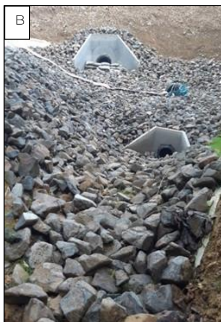
Plate 3-5: A) Stream at Site F1, upstream from SH1 in December 2023, B) Stream at Site F1 after construction in April 2024.
