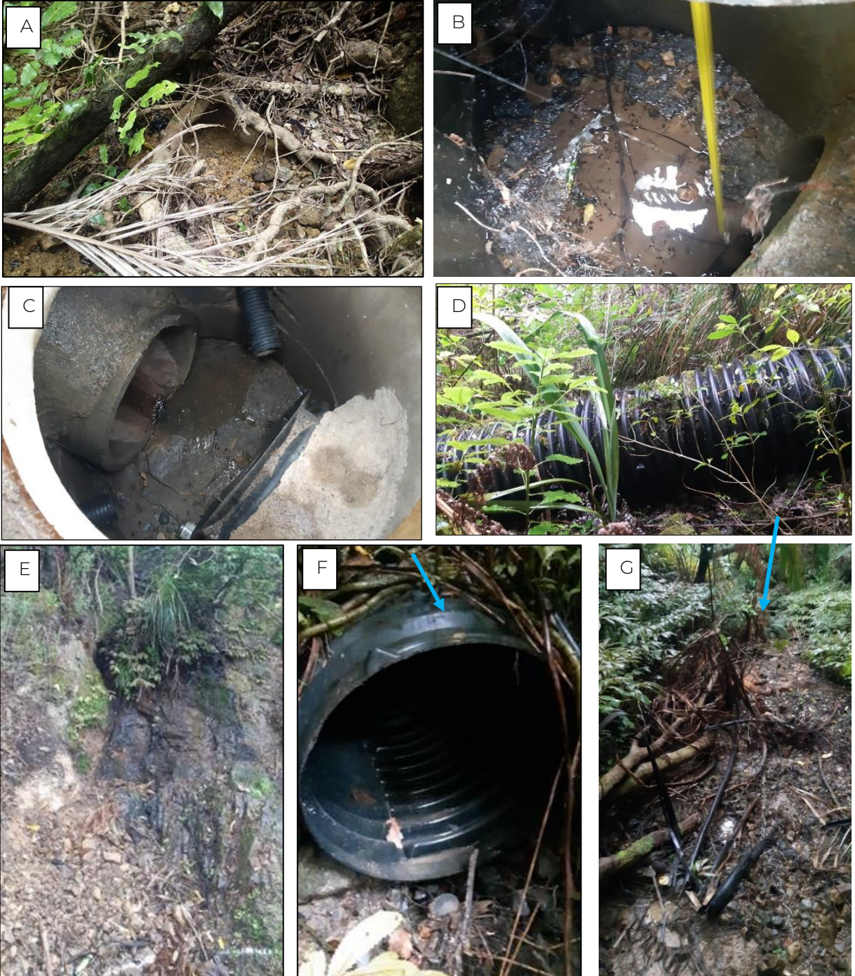
Plate 3-7: A) Stream at Site G3, upstream of SH1 in December 2023, B) Manhole upstream of the road with drop into inlet, C) manhole downstream of the road with flow disappearing before it flows down the flume, D) Flume down to stream, E) Stream at Site G3 upstream of SH1 in April 2024, F) perched outlet at end of flume, G) flows going subsurface at outlet of flume.
