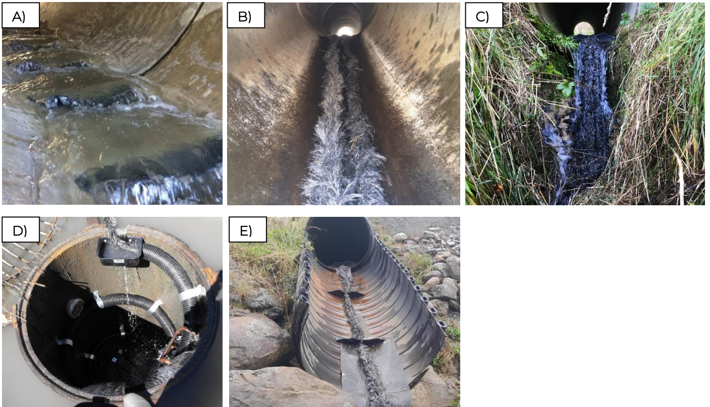
Figure A1. Low cost retrofit fish passage solutions A) baffles, B) mussel spat rope through culverts, C) mussel spat rope lined with PVC felt at outlets, D) combination of spat rope and pipe through manhole, E) spat rope and baffles through flume pipe.
