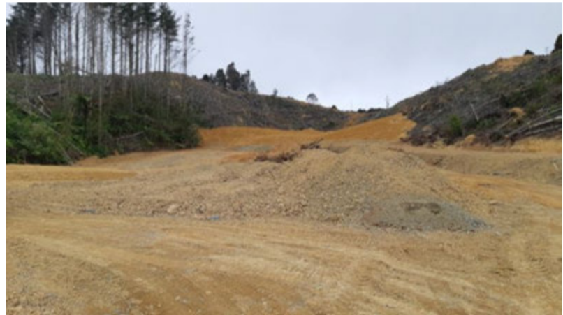
Photo 16: Site B1 Upstream: The wetland complex and stream during construction in April 2024. This has been completely reclaimed by fill area B.
