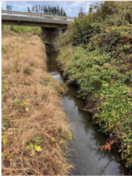
Photo 11: Site Piroa Stream Quarry: Stream habitat upstream of the road bridge within Atlas Quarry. The riparian vegetation was removed and a temporary culvert was installed.
