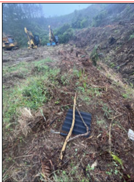
Photo 2: Site A Upstream: Section of stream upstream of the road during construction in December 2023. This section of stream was completely reclaimed by fill area A.
