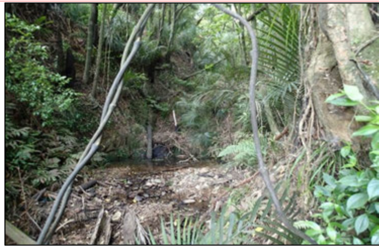
Photo 10: Site J: Stream habitat upstream of the road during construction in April 2024. Part of the section of stream was modified with a pipe extension and placement of rip rap.
