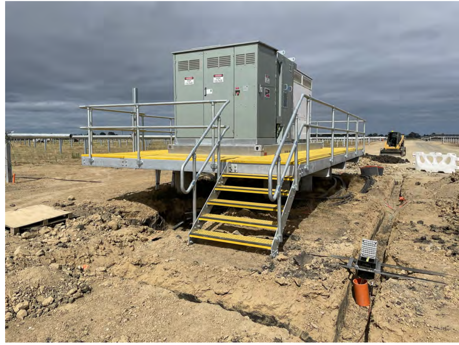
INDICATIVE POWER INVERTER STATION
