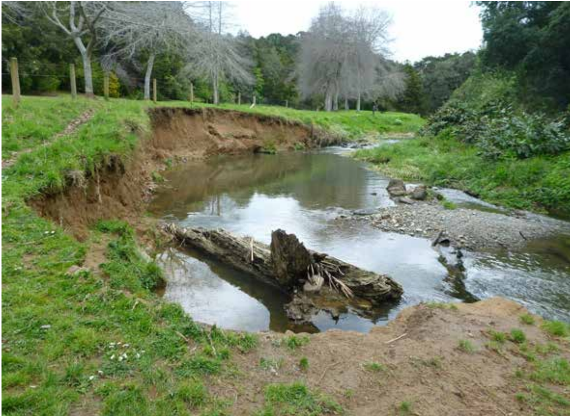
Erosion on the edge of a streambank – the Soil Conservation Strategy was developed by NRC in 2023 to help inform council's future response to erosion and sediment issues.
