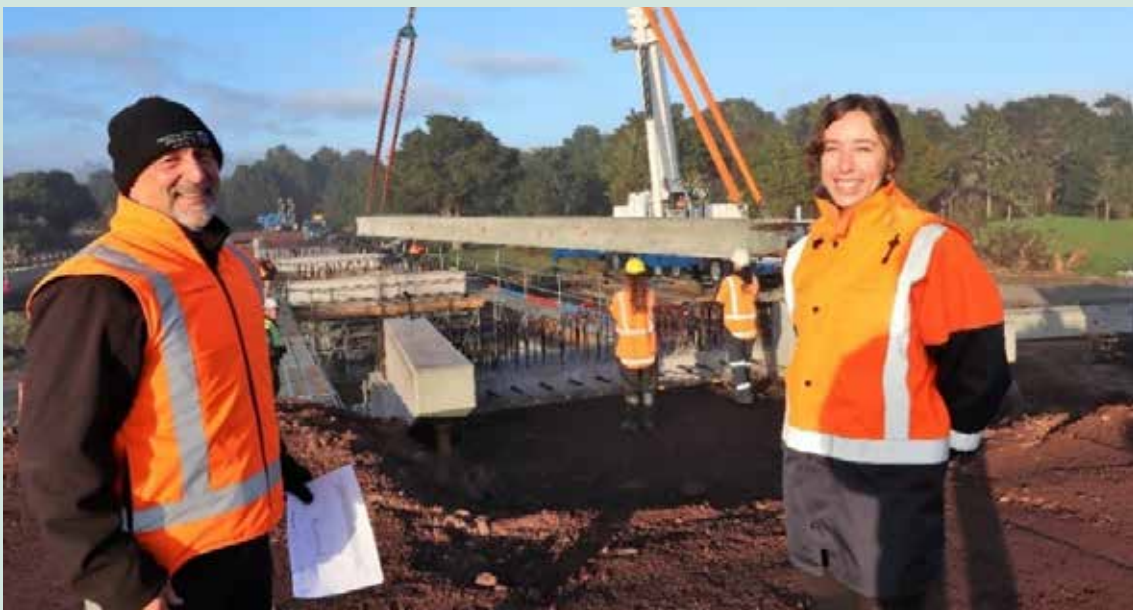
Construction of the new Pokapū Road bridge in Ōtiria, Northland. Source: https://www.nrc.govt.nz/news/2023/july/new-bridge-beams-in-place-as-part-of-otiria-moerewa-floodworks/
