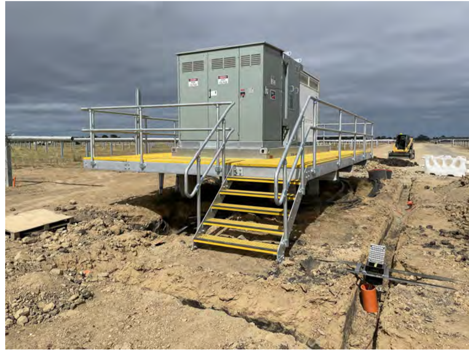
INDICATIVE POWER INVERTER STATION
