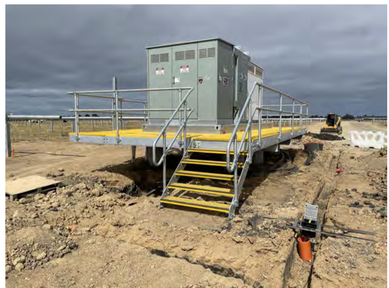
INDICATIVE POWER INVERTER STATION
