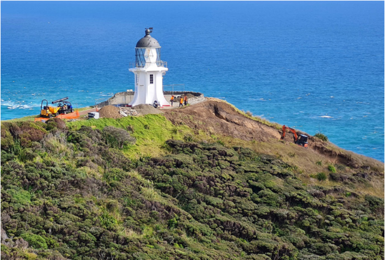
Rockwall collapse and slip at Te Rerenga Wairua | Cape Reinga, Ngāti Kuri rohe
