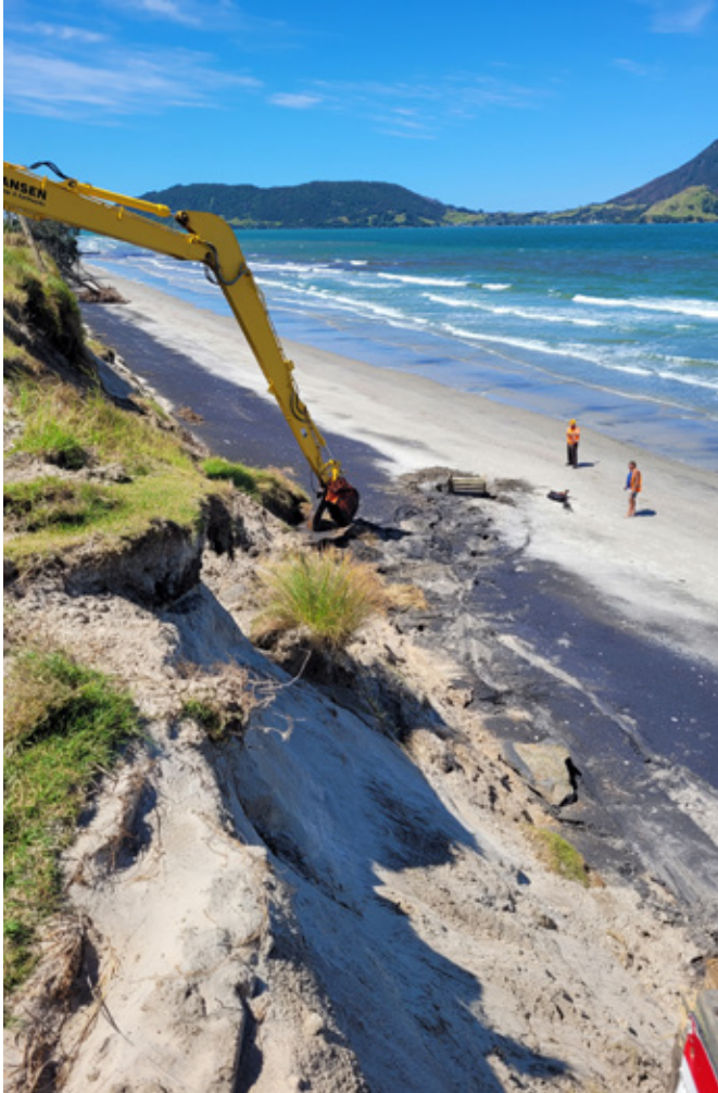
Coastal erosion and remedial works at Uretiti
