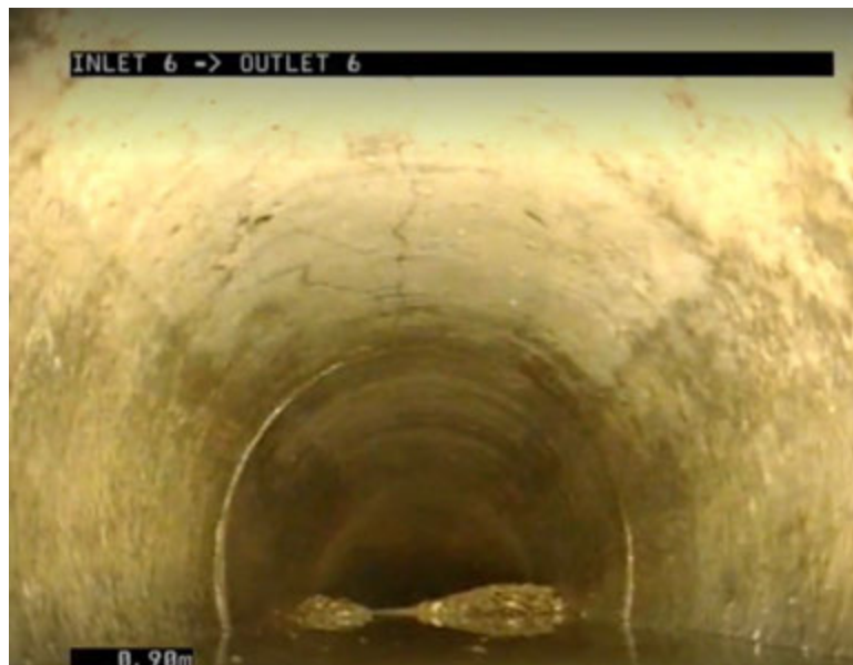
Figure 7 Culvert 12672 pipe has blockage (>30% Pipe Capacity)
